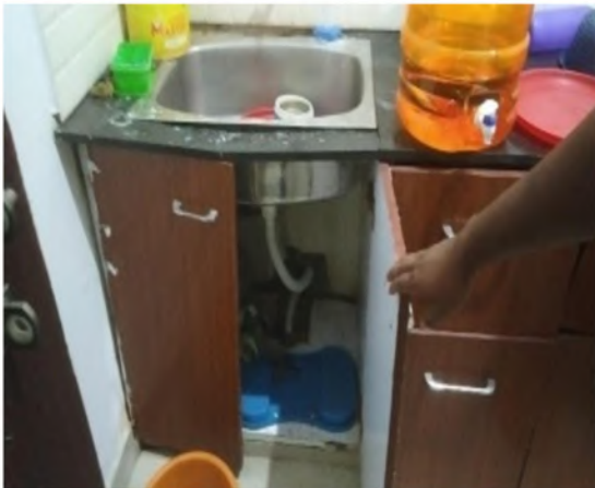
Damaged Kitchen Sink and Wood Work Kurugodu Police Quarters
