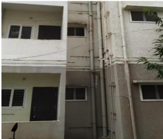
Poor Drainage System Yalanduru Police Quarters
