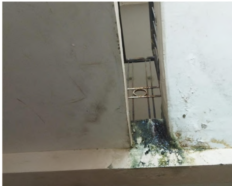
Figure 91: Water leakage leading to building damage in Chittapura Fire Station
