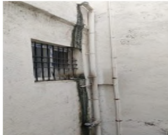
Seeping Pipes Shiraguppa Police Quarters
