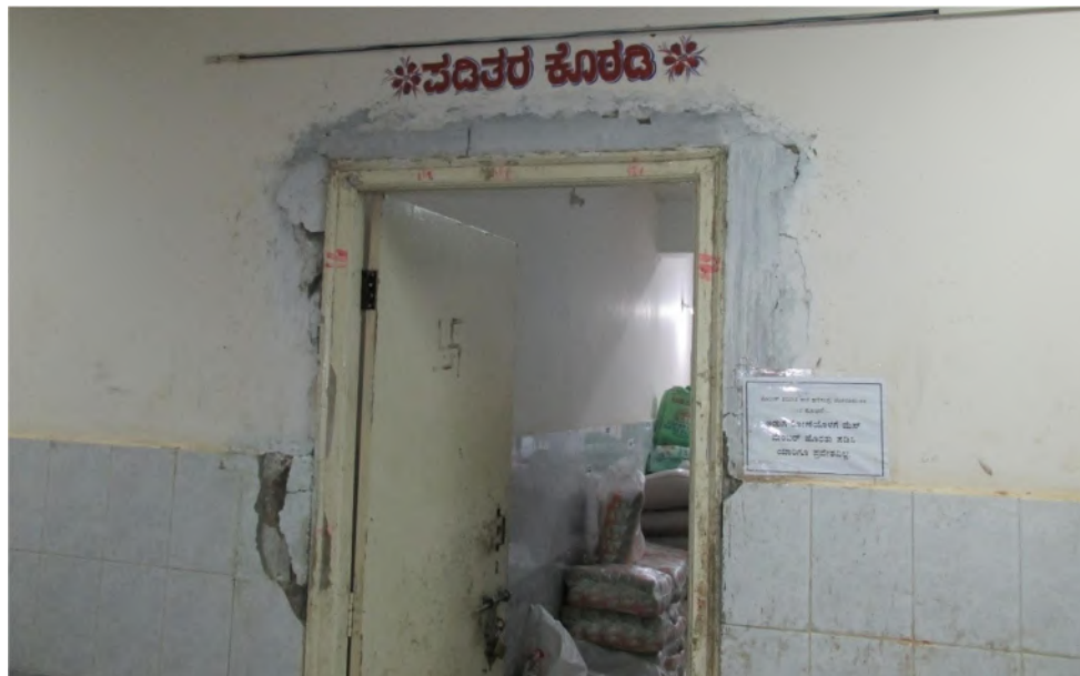
Figure 95: Crumbling walls in the Dining Block of PTS, Thanisandra
