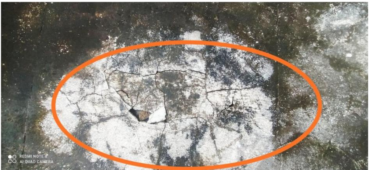
Figure 93: Cracked walls due to excessive seepage at Sulya Fire station
