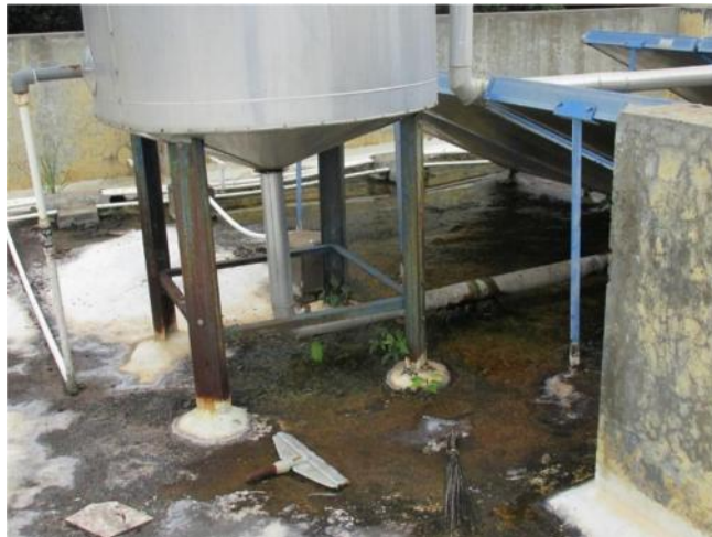
Figure 97: Poor maintenance of solar water heaters at Yelahanka PDMS Training and Hostel
