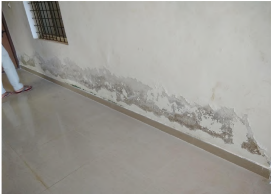
Figure 89: Poor quality of construction leading to seepage of water in the common areas at Chikkaballapura Fire Station
