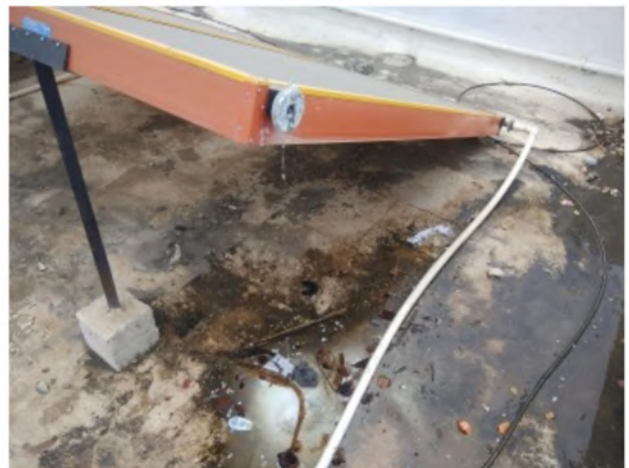
Poor Maintenance of Solar Water Panels
