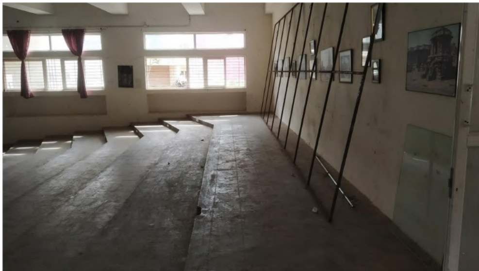
Figure 87: Poor maintenance of the auditorium
