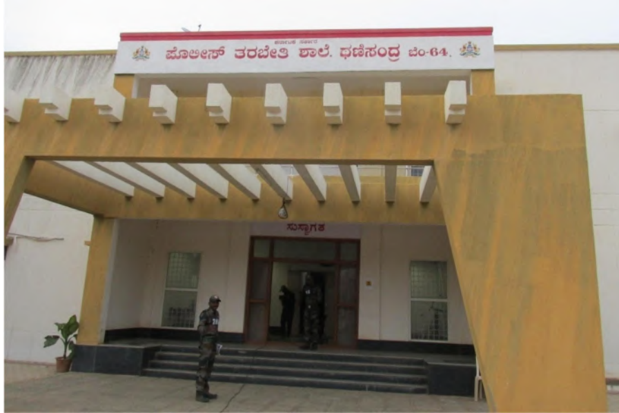
Figure 94: Faded front wall of the Administrative Block of PTS, Thanisandra
