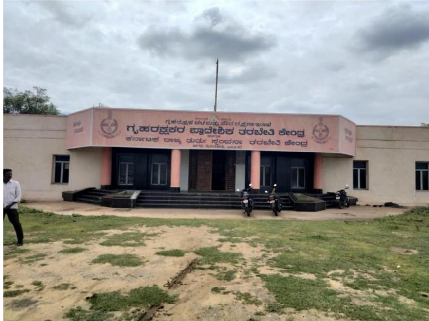
Figure 99: Lack of maintenance at DYSP Building
