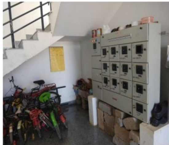
Open Electrical Panels without Safety Guards in Corridors
