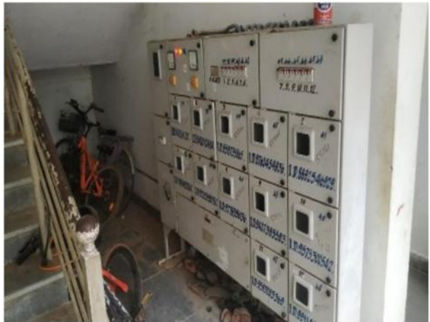
Open Electrical Panels
