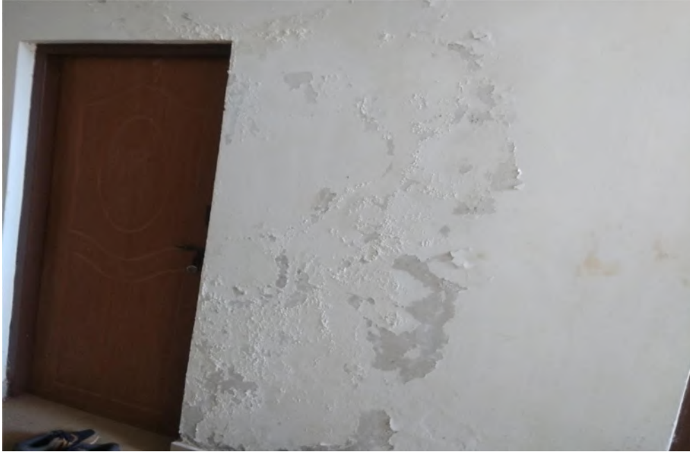
Figure 88: Poor quality of construction leading to seepage of water into the walls at Chikkaballapura Fire Station
