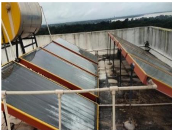
Poor Maintenance–Solar Water Panels
