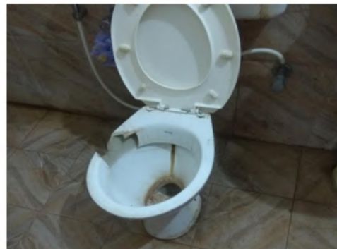
Broken Sanitary Ware – Binny Mills Police Housing Colony
