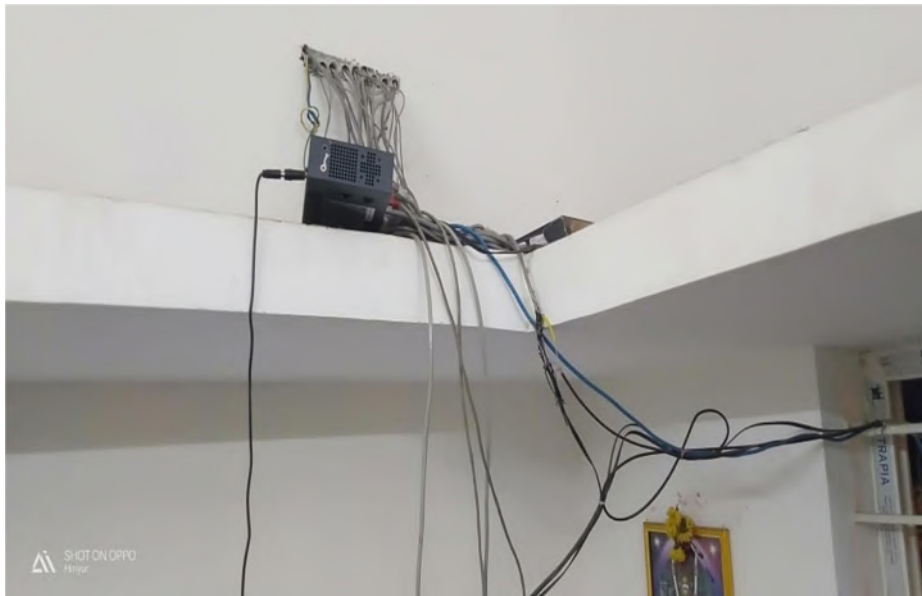
Figure 100: Poor electrical works at Hiriyyur Police Station
