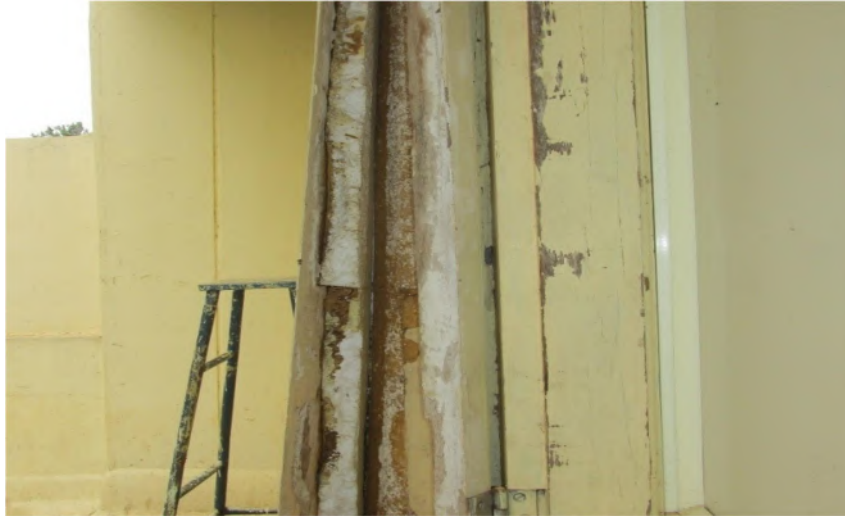
Figure 96: Poor Quality doors at PDMS Training and Hostel, Yelahanka
