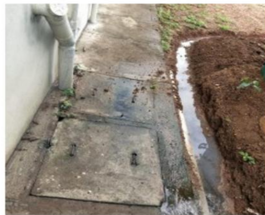
Poor & Improper Drainage
