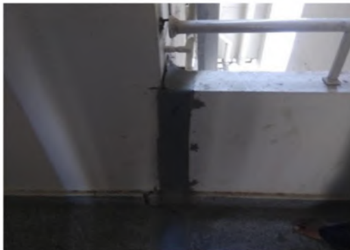
Cracks in Walls–Binny Mills Police Housing Colony
