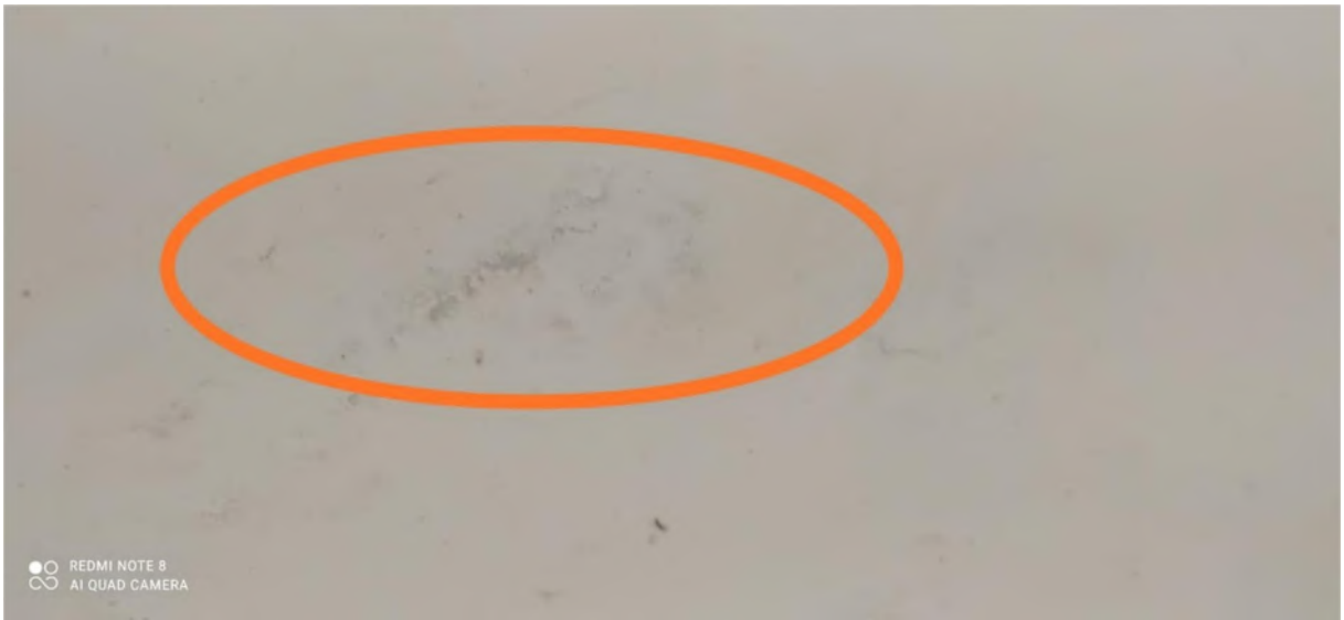
Figure 92: Water seepage through the ceiling at Sulya Fire station
