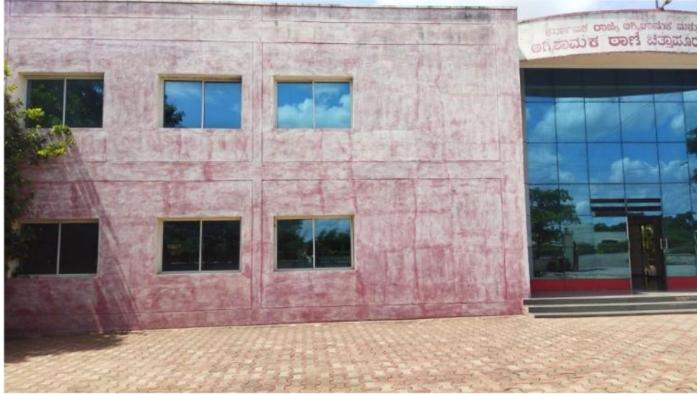
Figure 90: Poor quality of paint used for the external in Chittapura Fire Station
