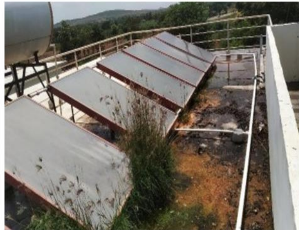
Poor Maintenance of Solar Water Panels Hanuru Police Quarters
