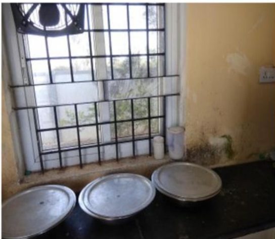
Poor Building Maintenance
